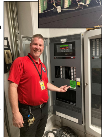
Top: Jail Access Controls Bottom: Green-Tag Fire System
